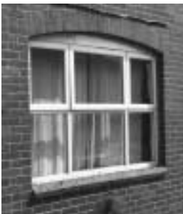
Incorrect construction using conventional DPC. Introduced in the first available horizontal run, this arrangement is suspect because it leaves a considerable amount of brickwork between window and DPC which is unprotected.
